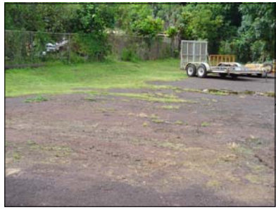
Drainage from the paved areas sheet flows to grassy or landscaped areas. Generally, storm water at the site sheet flows in the southwesterly direction, towards the southwest corner of the facility.
