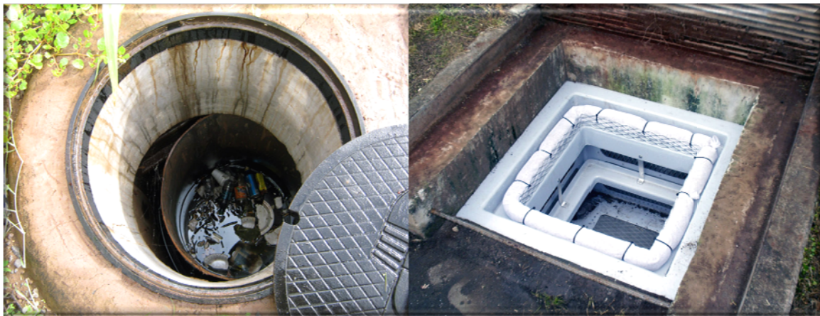
Hydrodynamic separators (left) and storm catch basin filter systems (right) trap trash, debris, and sediment before it can enter the MS4 and be discharged to the ocean.
