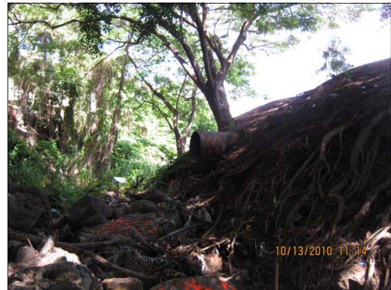
Photo 2: Outfall stream bank erosion
