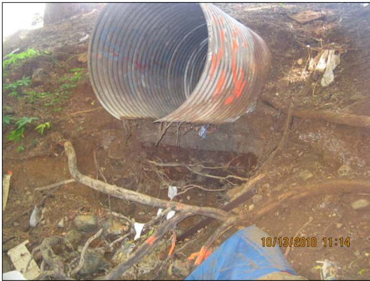
Photo 1: Corroded CMP outfall
