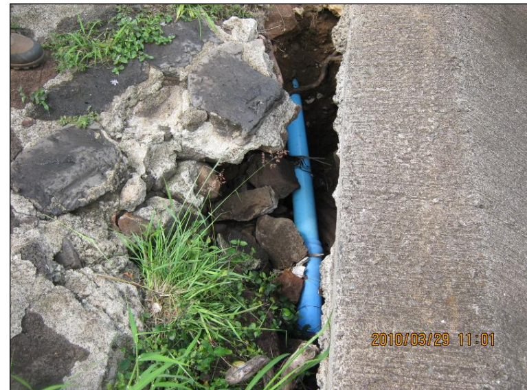
Photo 2: Eroded area behind concrete liner
