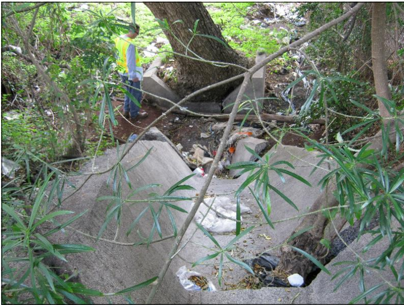
Photo 1: Failing concrete liner at outfall
