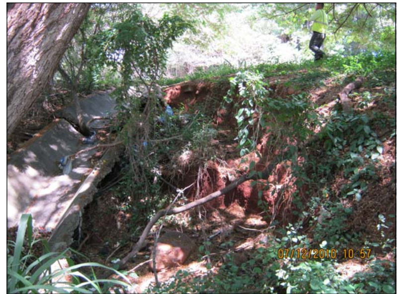
Photo 2: Erosion at outfall
