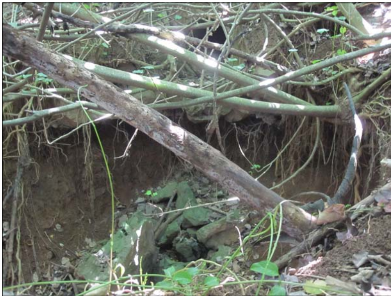
Photo 1: Undercut headwall and apron
