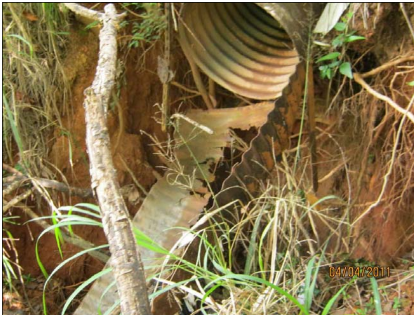
Photo 1: Pipe undermined due to erosion
