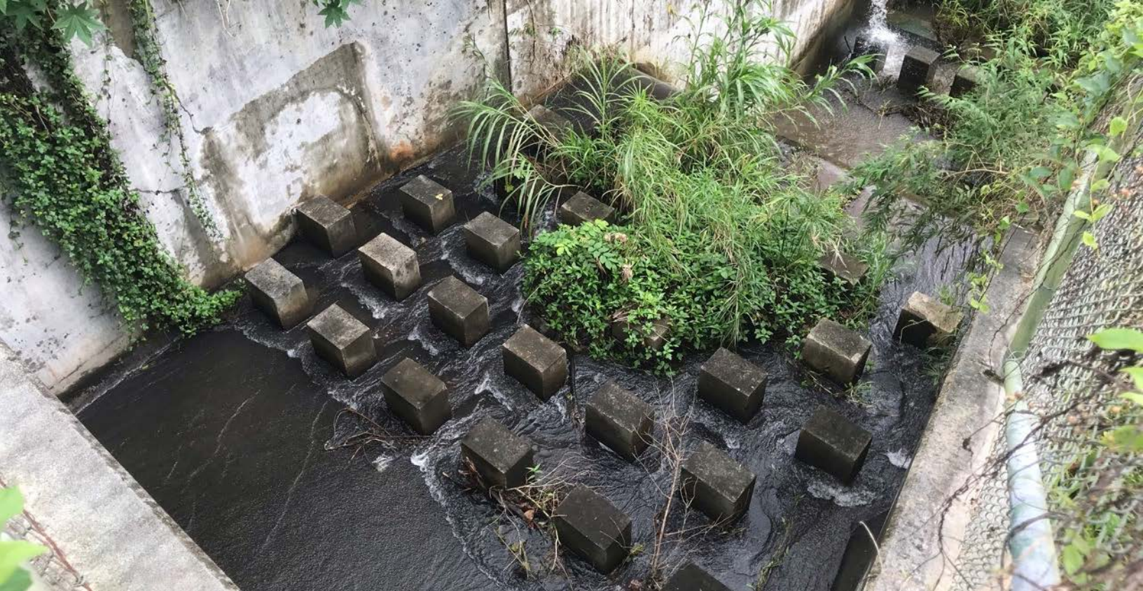
A drainage channel conveys storm water runoff on Pookela Street, Kaneohe, Hawaii.
