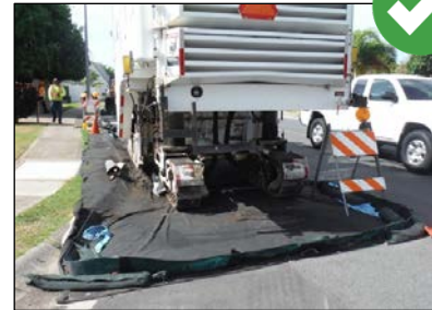
Idle paving equipment must be stored drip protection to contain leaks and spills.
