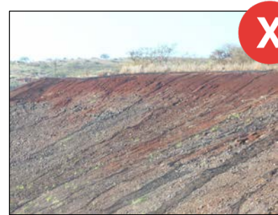
Additional mulch may be needed if erosion of hydroseeded area has occurred.
