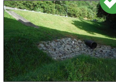
High flow velocities at the pipe outlet require the implementation of velocity dissipation devices to prevent downstream erosion.
