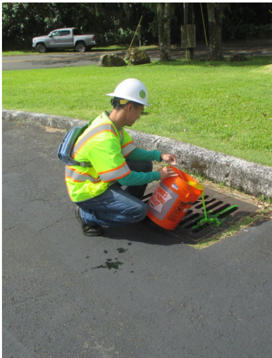
An inspector performs a dye test to verify the connectivity of the private drainage structure to the DOT-HWYS MS4.
