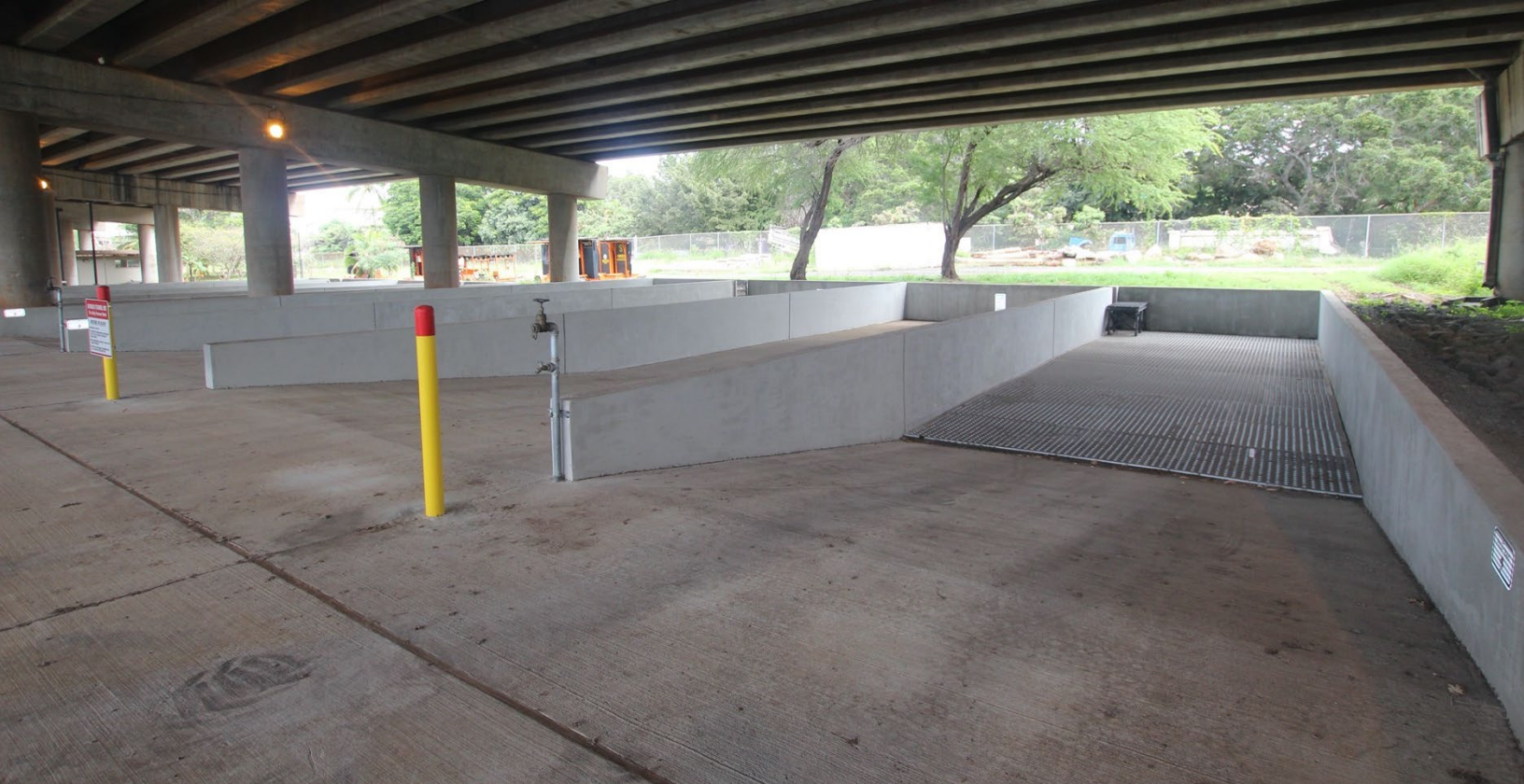
A Dewatering Facility is located at Pearl City Baseyard, Pearl City, Hawaii.
