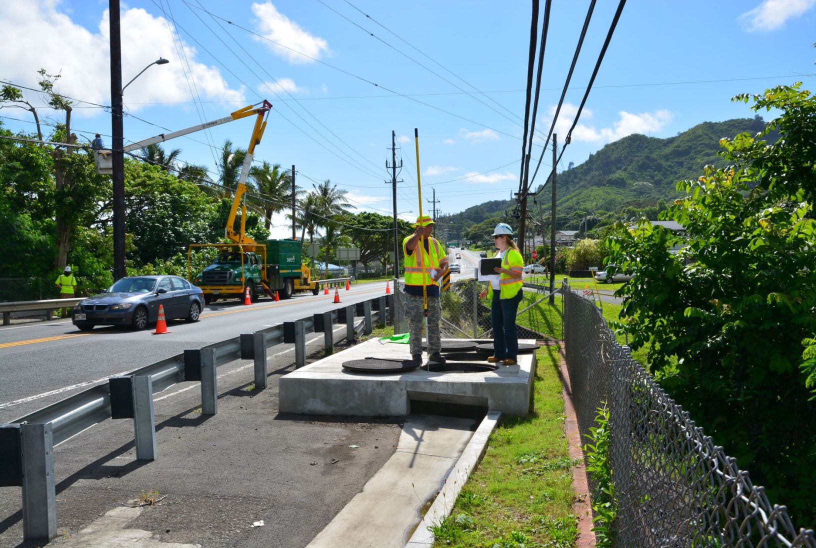
Inspectors collect grab samples from a water polisher along Kaneohe Bay Drive, Kaneohe, Hawaii.
