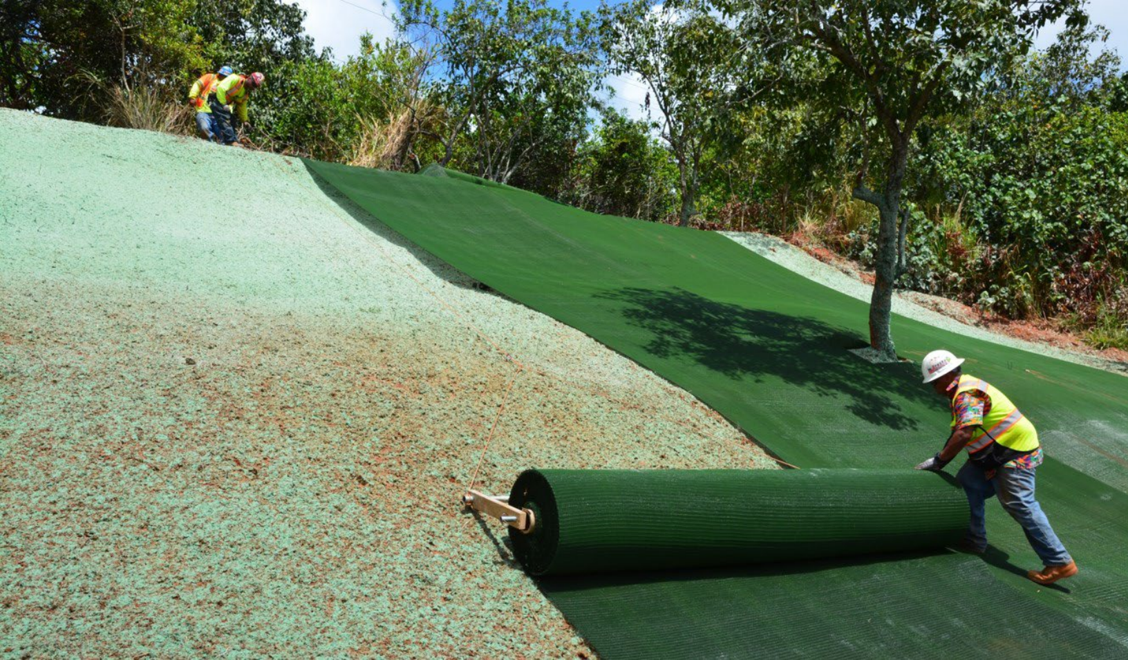
Eroded slope repair addresses sediment and nutrients loading along Kalanianaʻole Highway in Kailua, Hawaii.
