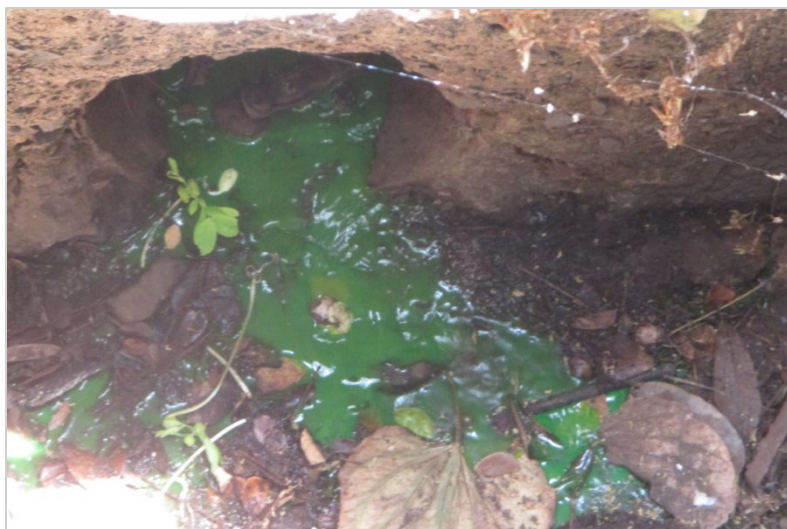
A dye test verifies the connectivity of a private drainage structure to the DOT-HWYS MS4.
