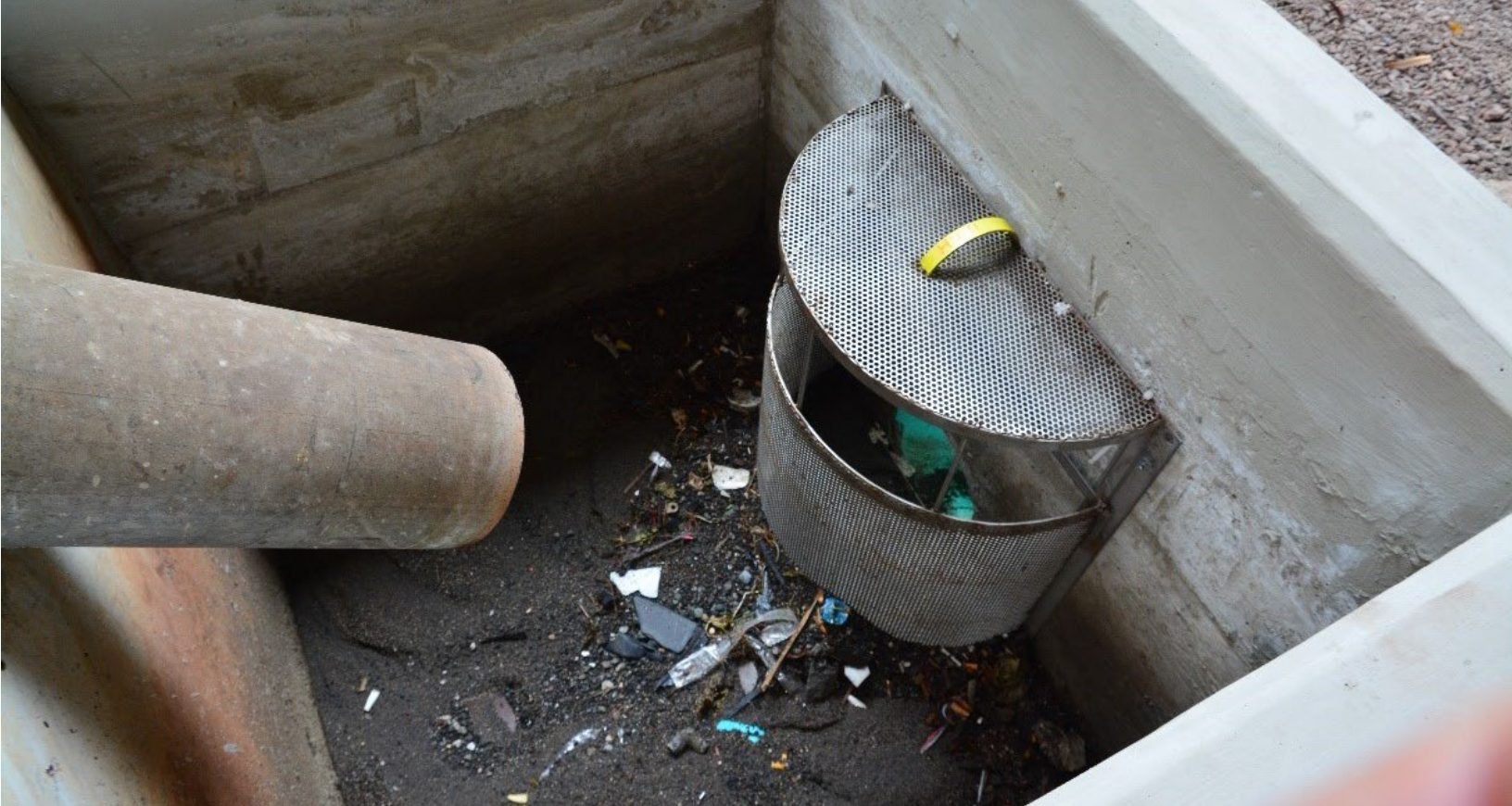
A downspout filter box captures pollutants under the H-1 Viaduct in the Waimalu Watershed.
