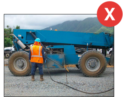
There must be drip protection under vehicles and equipment that are being refueled on-site.
