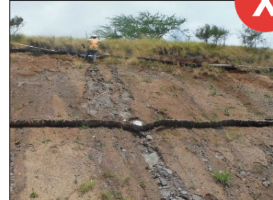
Compost filter berms that do not maintain direct contact with soil allows erosion and undermining to occur.
