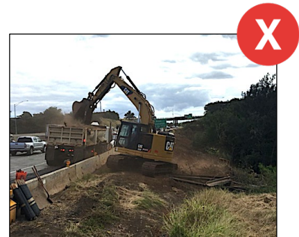
Not using dust control measures can result in excessive dust being generated by construction activities.
