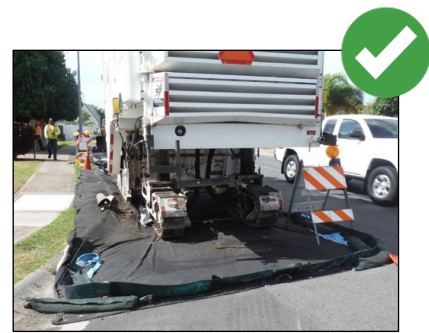
Idle paving equipment must be stored drip protection to contain leaks and spills.
