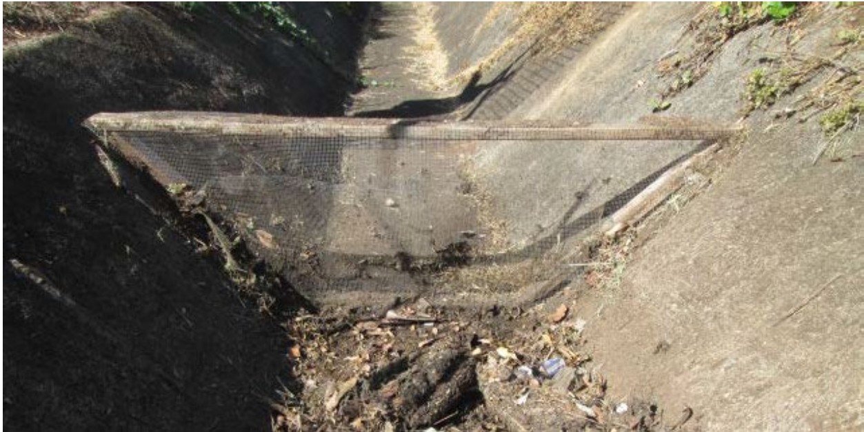
Figure 4. Trash trap located at Site #3.
