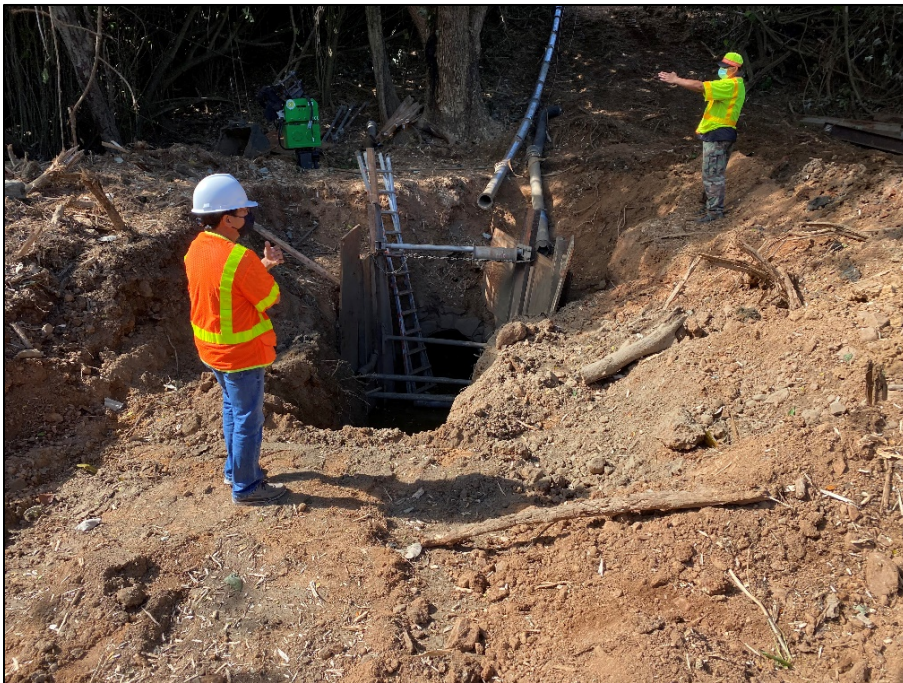
Sedimentation at outfall
