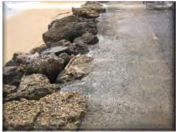
Tidal sand on the road.
