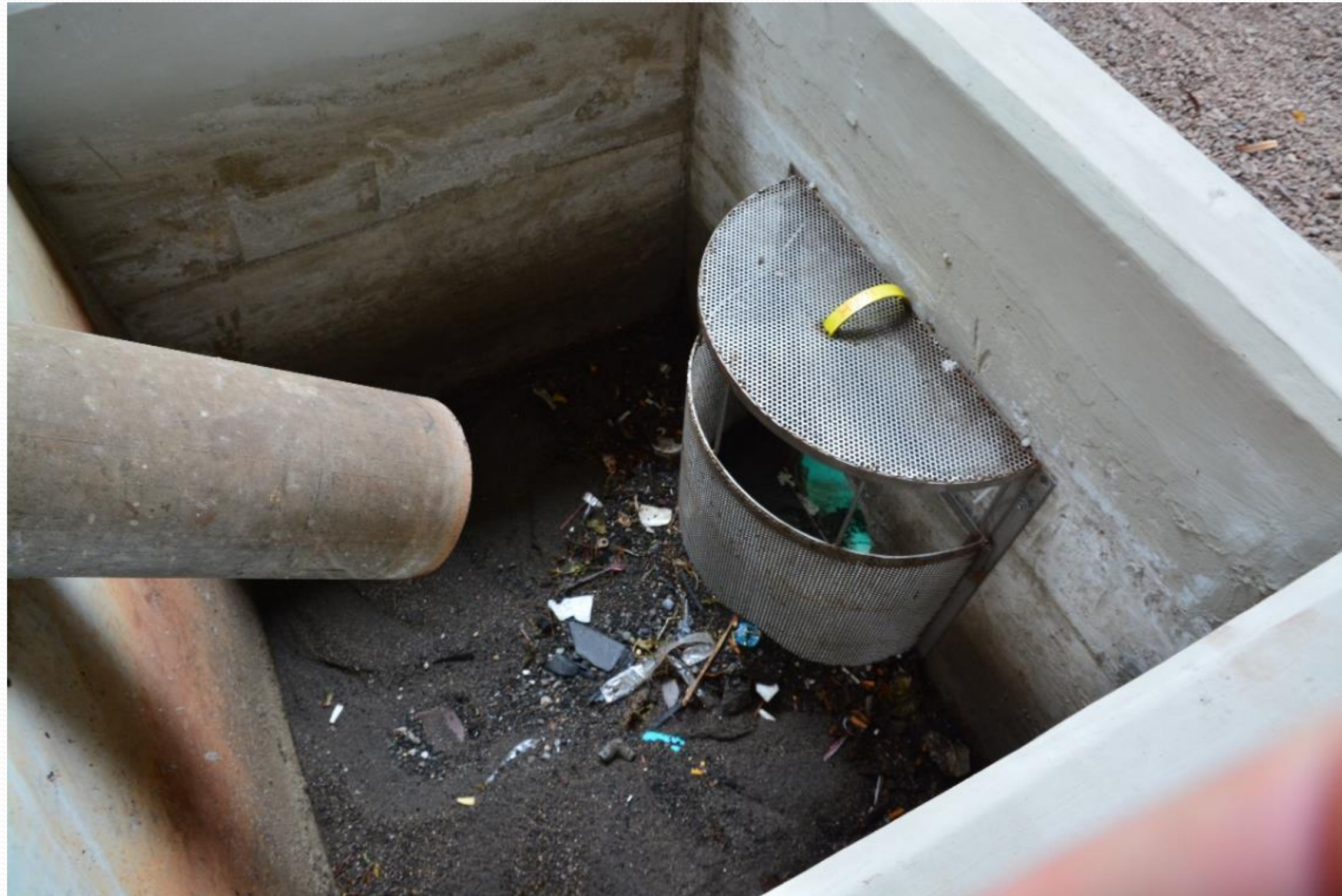
Downspout Filter Box
